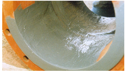
The daily repair routine when epoxy ceramic compounds are used for linings. No hydraulic engineer wants to see irregular surfaces like this ...
